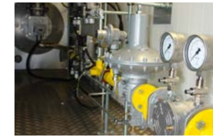
Gas control valves inside a TURBO
