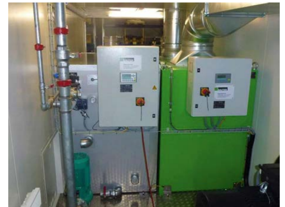
OLH installed beside a HWS inside a container
