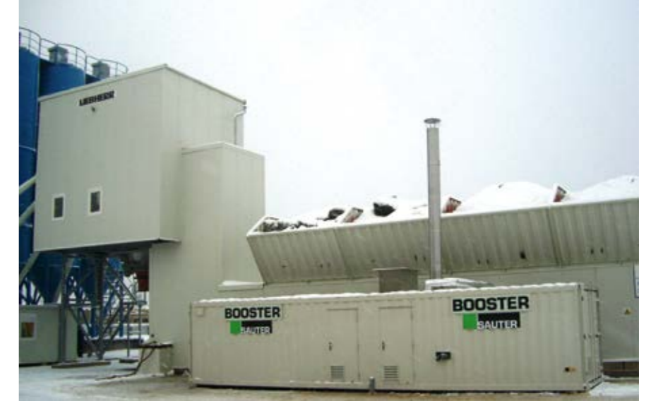
Containerized BOOSTER systems under harsh climatic conditions
